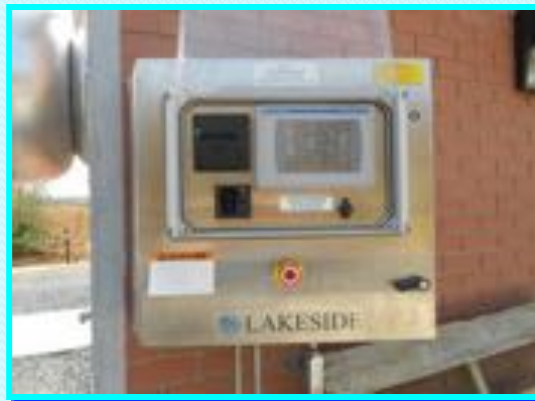
Access Control System
