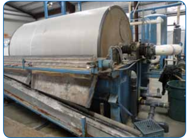
Alar dewatering system, Sierra Septic Treatment Facility.
